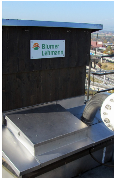
grit silo plant with gritting vehicles in Bern Wankdorf
